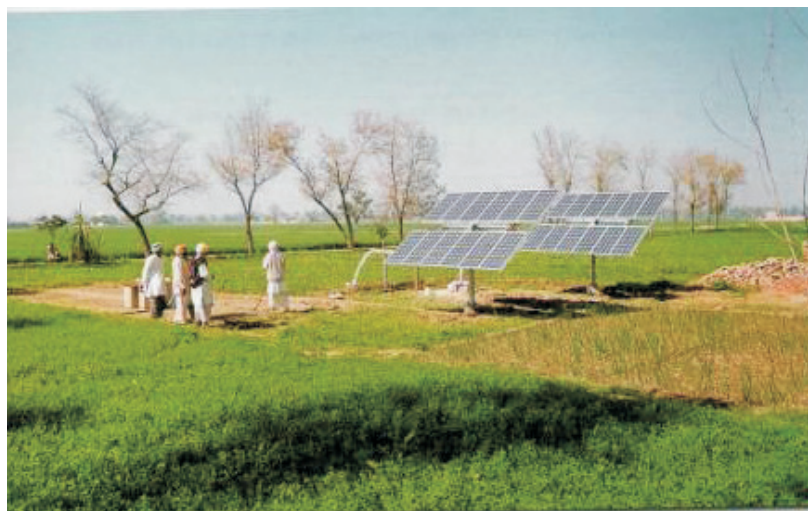
Fig. 12.2 Photovoltaic Water Pumping
